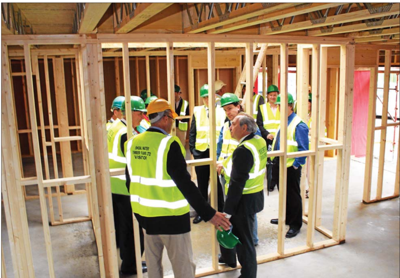
(p33) The country's first commercial passive house development in Rosslare is built using Irish products and Irish expertise, with traditional Irish design features; (above, left) the timber frame system was manufactured and erected by Shoalwater Timber frame; (middle and right) they were also responsible for the airtightness of the house and used the ProClima system of membranes, tapes and adhesives; (p37) windows are triple-glazed from Munster Joinery and are the first Irish products to undergo testing for Passive House Institute certification
